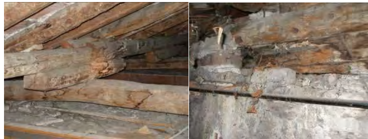
Figure 50_ – Water leakages on the wooden beams of the roof.
