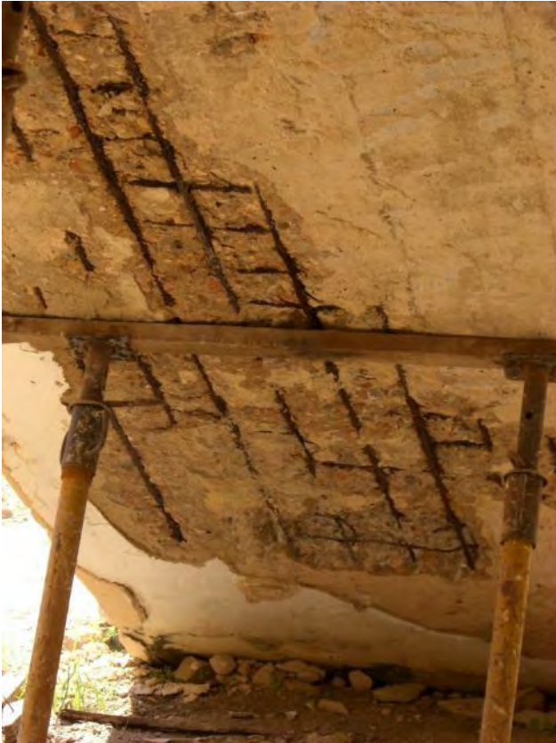
Figura 24_ Degraded concrete slabs
