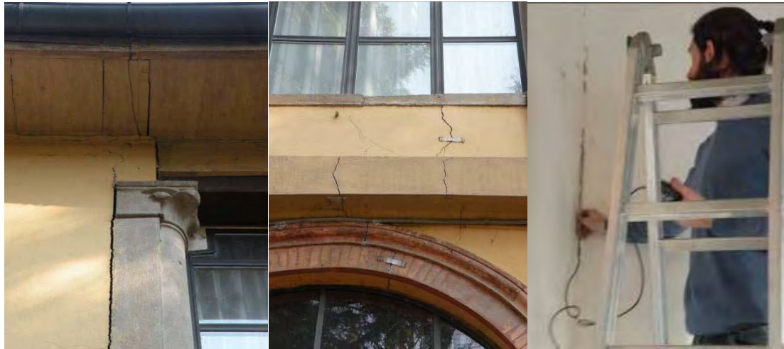
Figure 47_ Cracks on the exterior walls in the SW side (left and centre); measurement of the air-flow through cracks from the interior with an anemometer (right)
