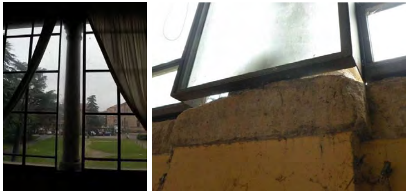
Figure 53_Window frame around a masonry column (left) and detail of the opening (right), 1st floor, front side of the building.
