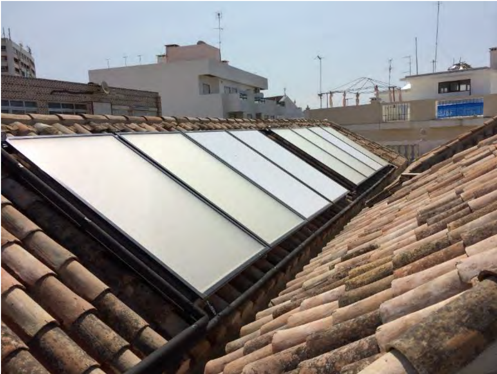
Figure 32_ Solar panels on the roof
