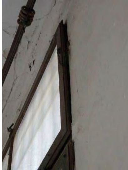
Figure 55_Detail of a window of the ground floor with a “bad closing”.
