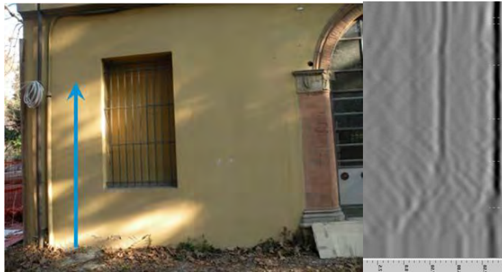
Figure 51_GPR radar for moisture detection: vertical survey line on a masonry wall (left) and the collected radargram (right).
