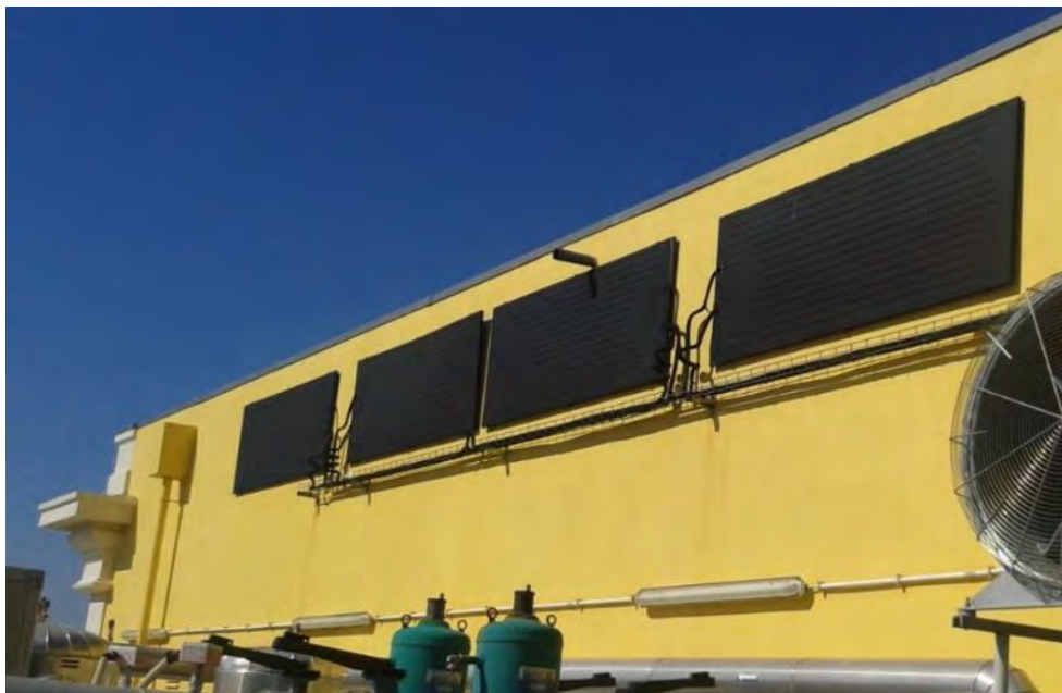
Figure 16_ Solar panels of Cineteatro Louletano
