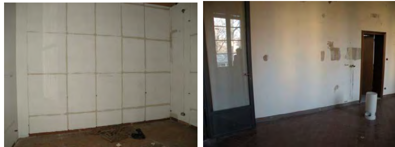
Figure 35_Vertical opaque walls in the ground floor (top) and 1st floor (bottom)
